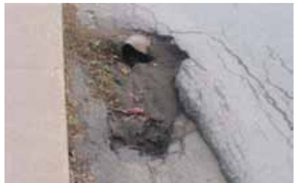
Figure 3. Pothole near back entrance to Rite Aid.
