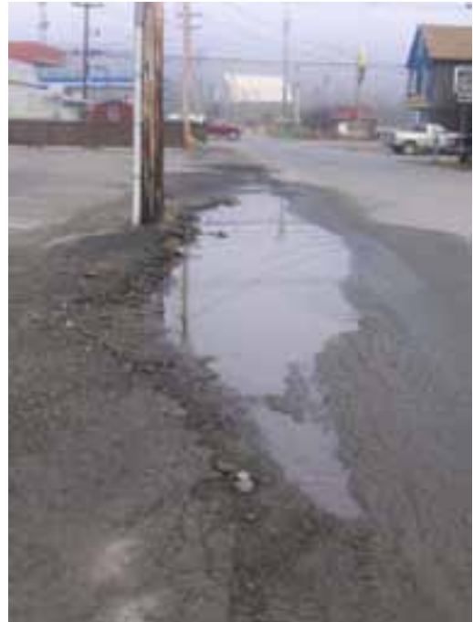
Figure 2. Section of road in front of cinema needing repair.
